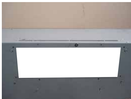
Horizontal Ducting (3-1/4"x10" Rectangular)
