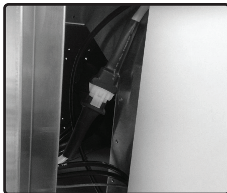
8. Connect 6 pin molex connector from capacitor cable to 6 pin molex connector from control box. Connect 2 pin plug from AC power cable to 2 pin plug from control box. Secure cables to hood interior with zip ties and zip tie holders.
