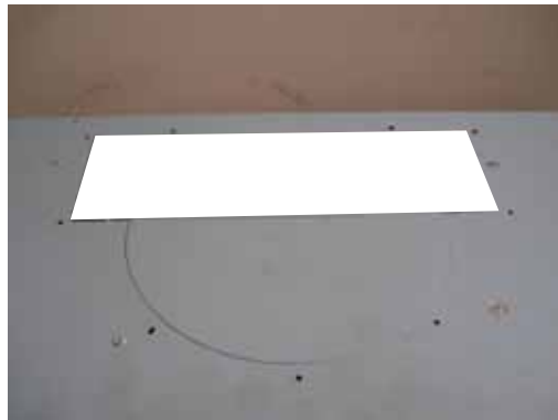
Vertical Ducting (3-1/4"x10" Rectangular)
